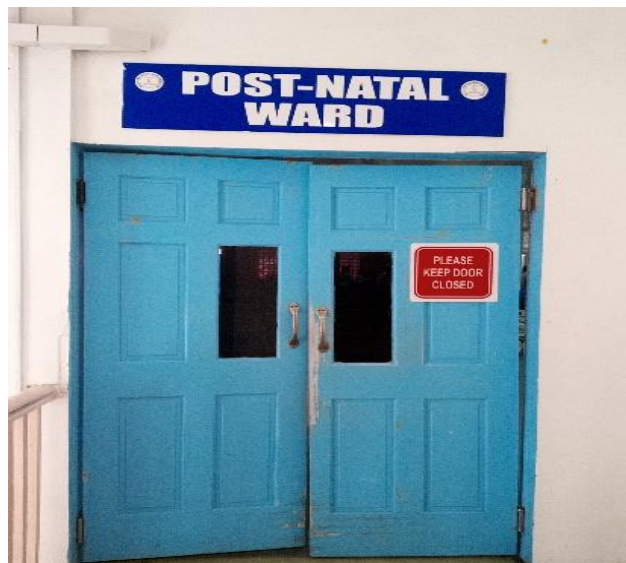
Figure 10 – Damaged door making it unable to be closed Source: Audit Office of Guyana — Date taken 2022/6/23
