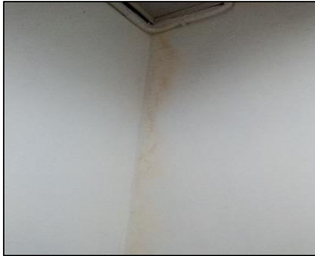
Figure 5 – Water stains from leaks in the Triage area of the Maternity Unit at GPHC
