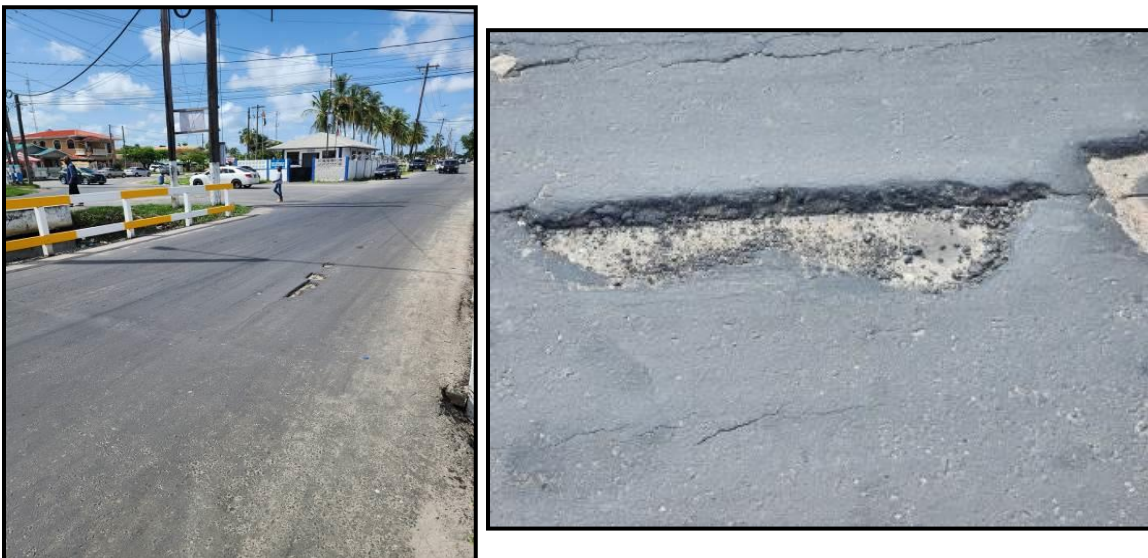
Photographs of the deteriorating asphalt overlay on timber bridge at Vlissengen Road (Between Princess Street and Mandela Avenue)- 15 August 2023
