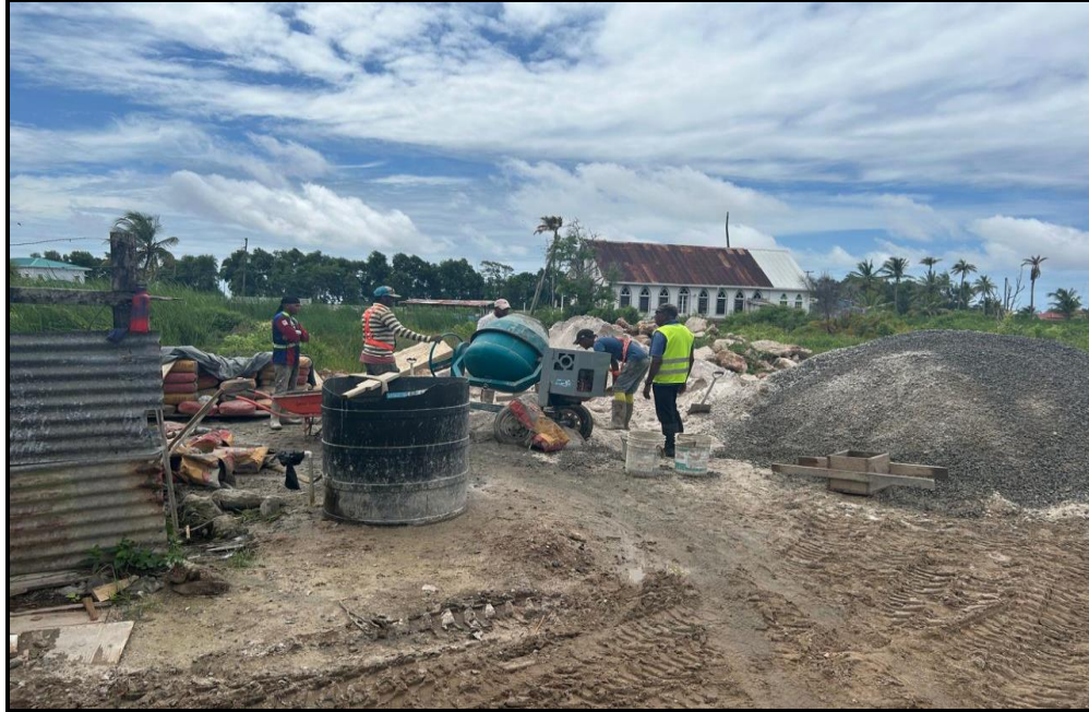
Photograph of grossly inaccurate, poor methodology and unacceptable batching of concrete observed on site during concrete pouring at Dorm Building, Mahaica Hospital - 13 June 2024
