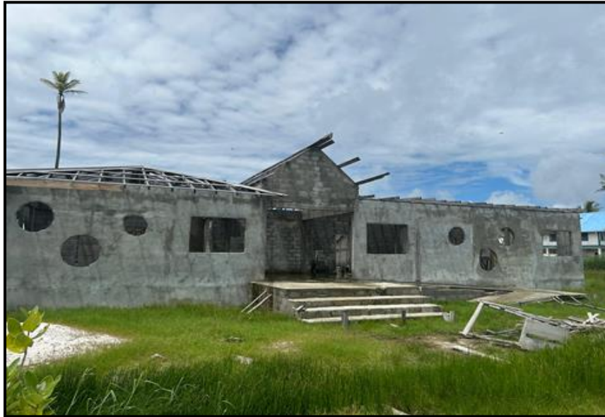
Photograph of the incomplete building at the Child Care Centre, Mahaica - 19 June 2024
