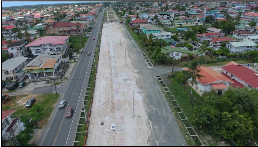
Photograph of the incomplete works at termination at Conversation Tree to Dennis Street- 15 August 2023
