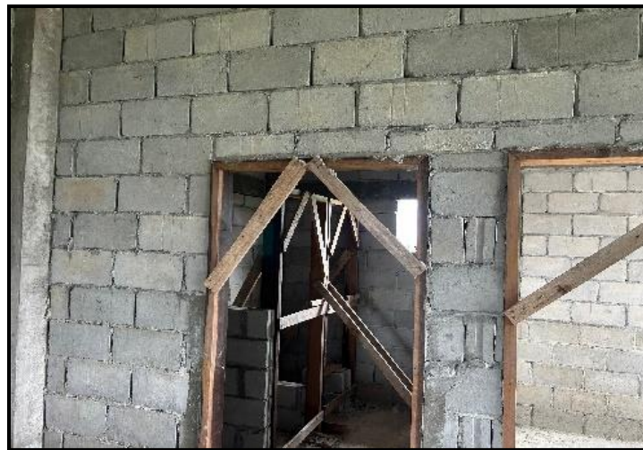
Photographs of no lintel beams above doors at the Day and Night Care Facility - 12 June 2024
