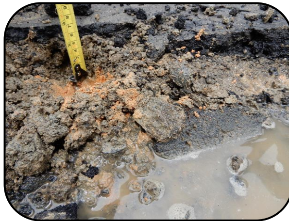
Photos of the defective works done
