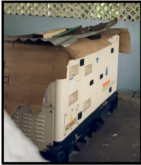
Photo of Generator at Long Creek Health Centre
