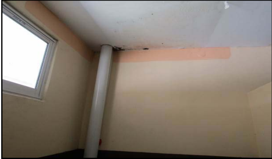
Leak observed on ceiling in washroom on the ground floor
