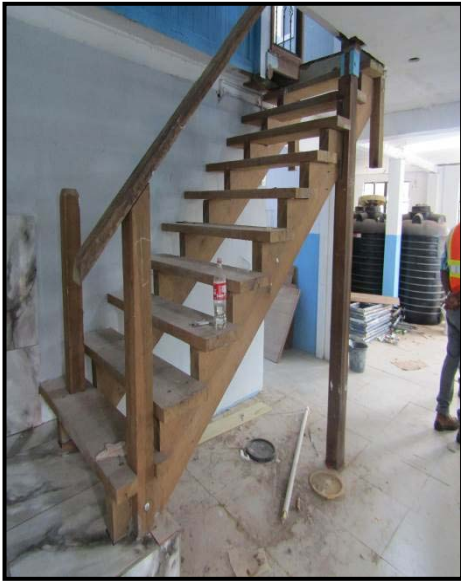
Lacquer not applied to stair case
