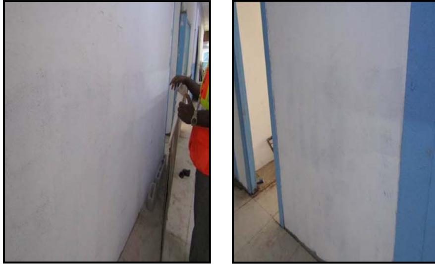
Poor quality of painting work observed
