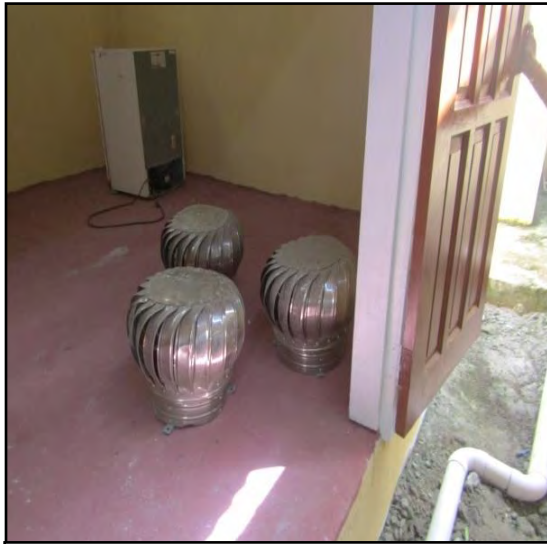
Extractor fans not installed but full payment issued to the Contractor
