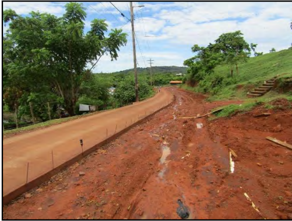
No reinforced concrete drains constructed and only half of the reinforced concrete payment completed
