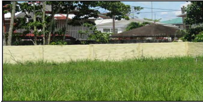
Shoddy rendering works completed to fence
