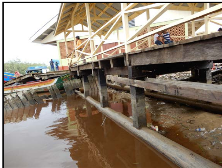
Wharf at Kumaka without ties to columns
