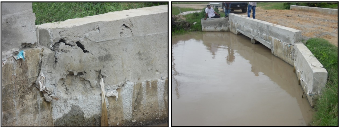
Poor quality concrete works
