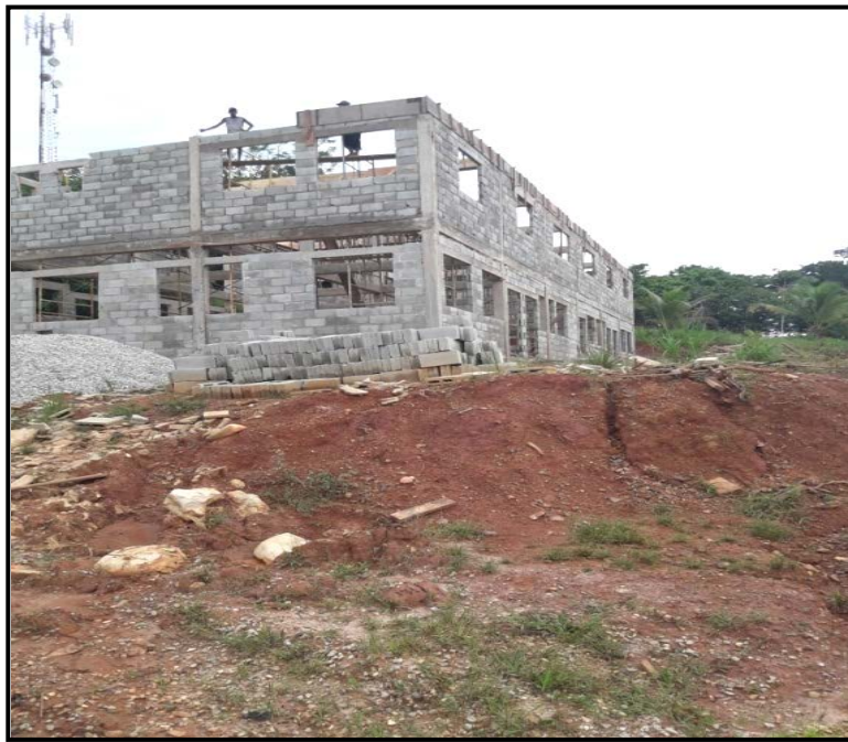
The works executed on the building (Photo taken on 30 August 2017, at the time of physical verification)
