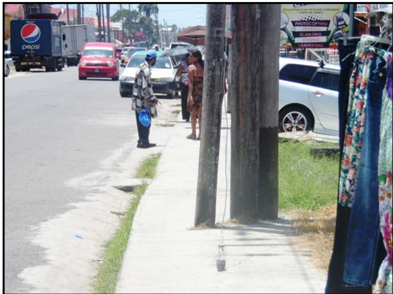
Completed walkway with GPL Poles and GWI Valve Chambers which were not relocated
