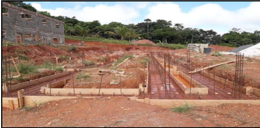
The works executed on the foundation-Photo taken on 30 August 2017, at the time of physical verification.
