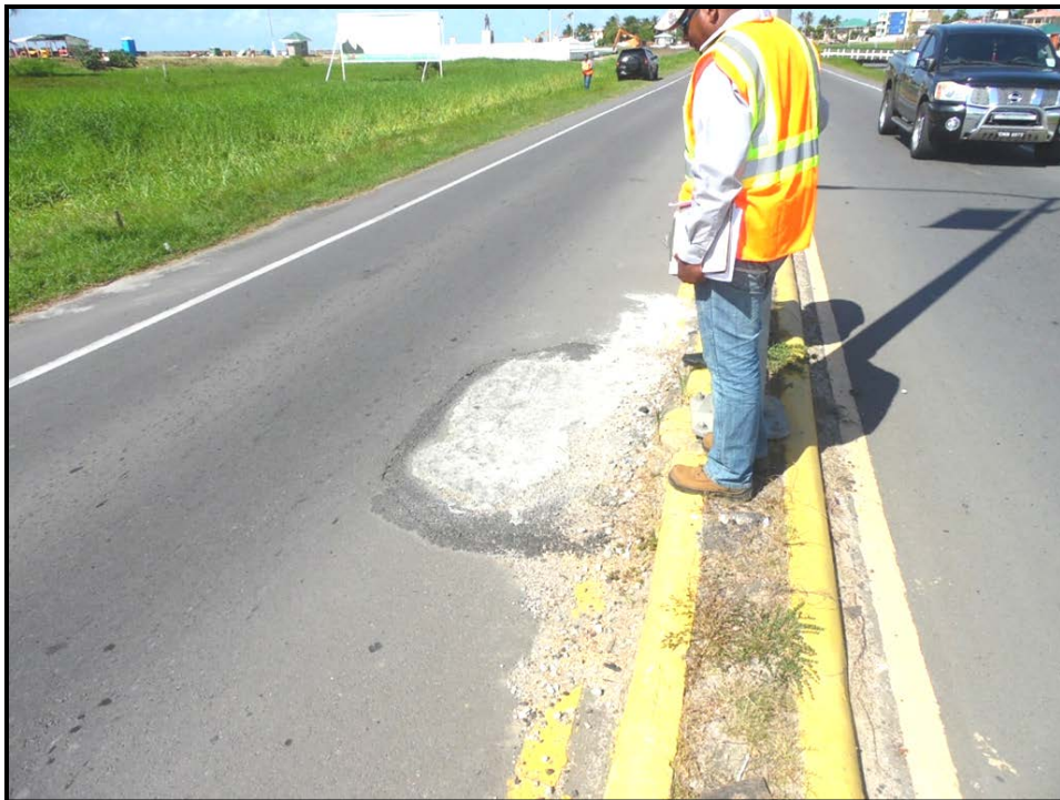
Depressions developing at the base of light poles along the roadway
